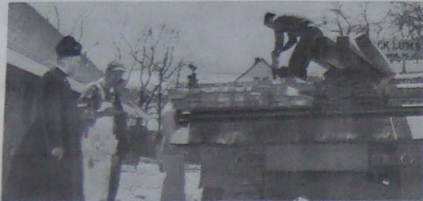
FATHER EUGENE F. SULLIVAN looks on as parish members unload lumber. "We have practically made up our own construction company from members of the parish and friends," says Father Sullivan.
