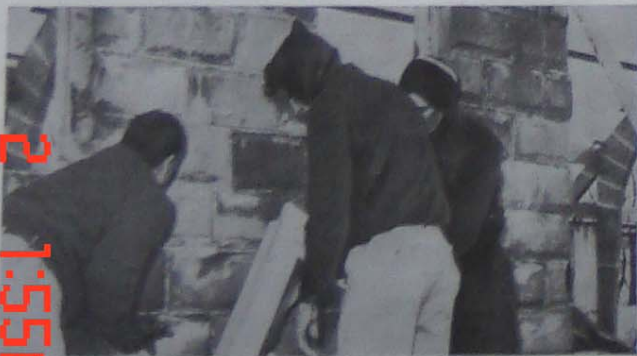
WORKING THE YEAR AROUND in all kinds of faiths have joined with their neighbors to construct first Catholic Church in Washington Township, N.J.
