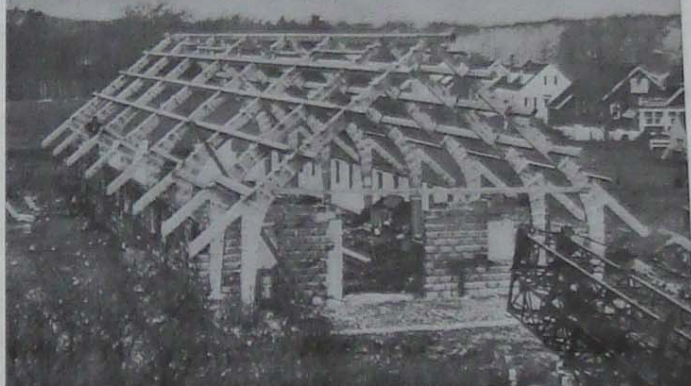
The framework of Our Lady of Good Counsel Church rises from barn ruins. Grounds have been cleared and leveled.
